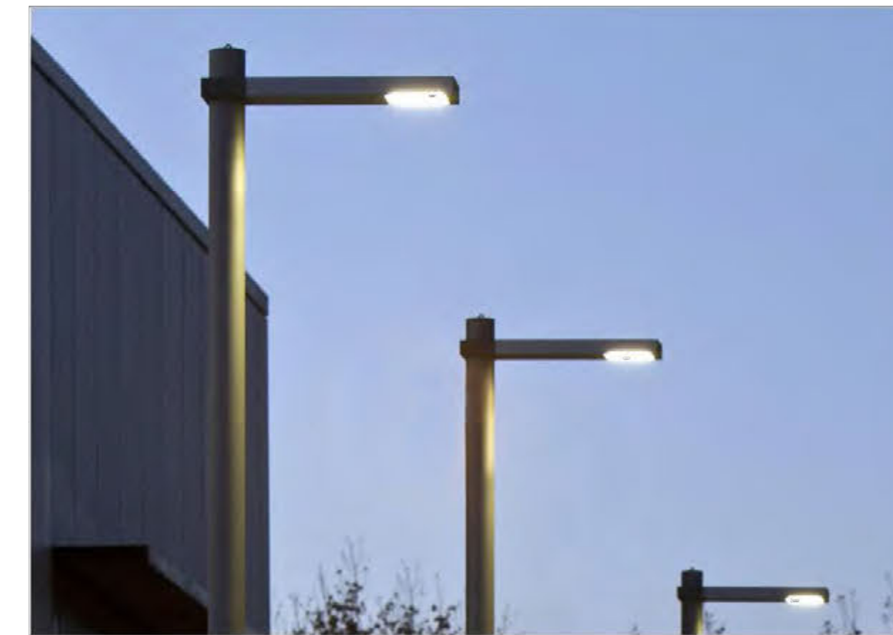
ROADWAY LIGHT FIXTURES
